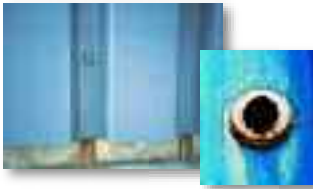
Loss of pull over value on the fastener head and unsightly rust stains due to corrosion of fastener
