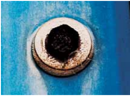
Corrosion of fastener head
