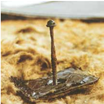
Coated carbon steel corrosion in a flat roofing fastener
