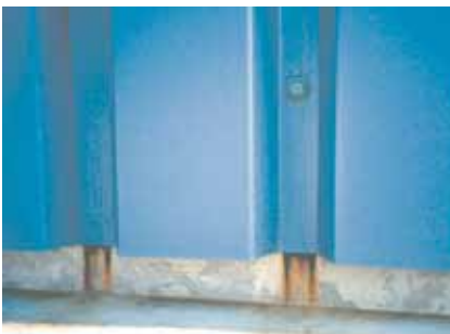
.....rust staining on cladding.....
